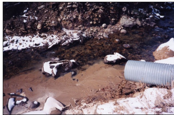
Figure 4. Nonpoint source pollution from the Lefthand OHV Area entering Lefthand Creek via a culvert under County Road 94.
